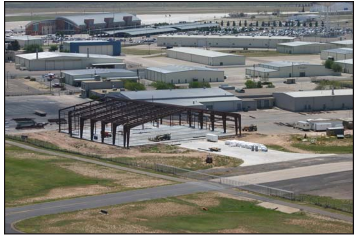
On our return to the airport, H.A. snapped this photo of the new Commemorative Center construction. Since then, even more of the building is in place as Col Ralph Gillette will report and show you at the meeting.
